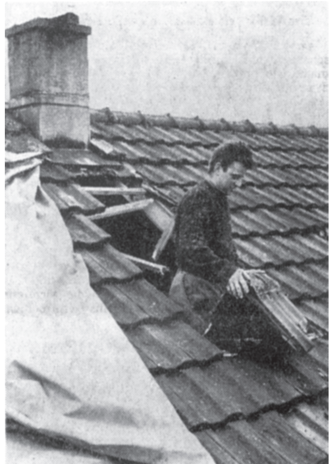
Fig. 7. Sarnen: The top of a chimney destroyed part of the roof (Vaterland, February 18, 1964)
