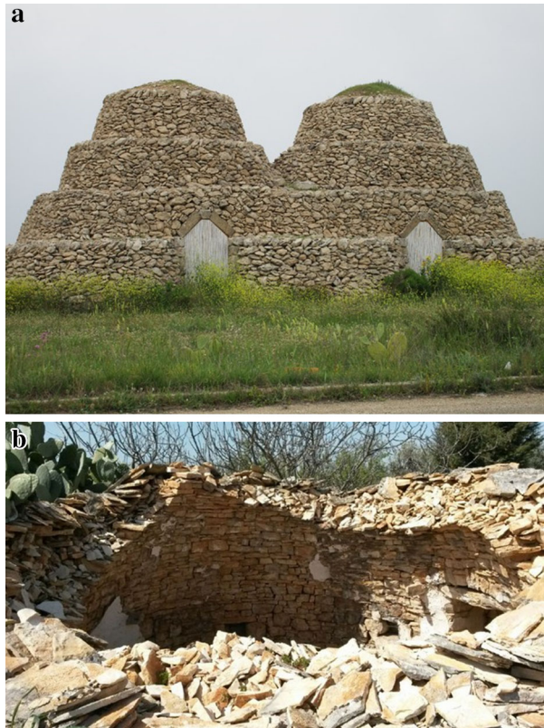
Fig. 4 Two examples of pagghiare, dry-stone vernacular constructions located at south of Apulia region. a external view of two pagghiare; b a cross-section of a pagghiara after its collapse
