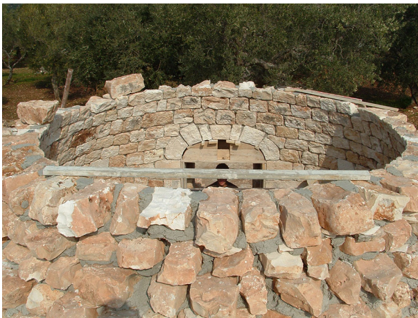
Fig. 11 Construction of the candela without centring: the inclusion of small stones ( scarde ) and/or, more recently, mortar guarantee the continuity of the horizontal rings
