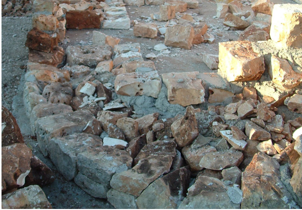
Fig. 7 Wall under construction. It consists of internal and external leaves of large and regular calcareous stones, with mortar poured between them
