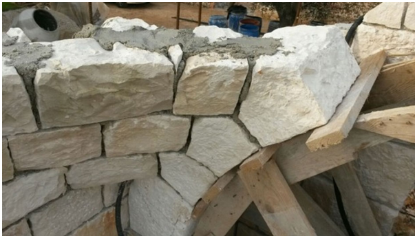
Fig. 10 Detail of a corner, where the stones comply with two different static paths: the arch and the pseudo-horizontal ring of the dome
