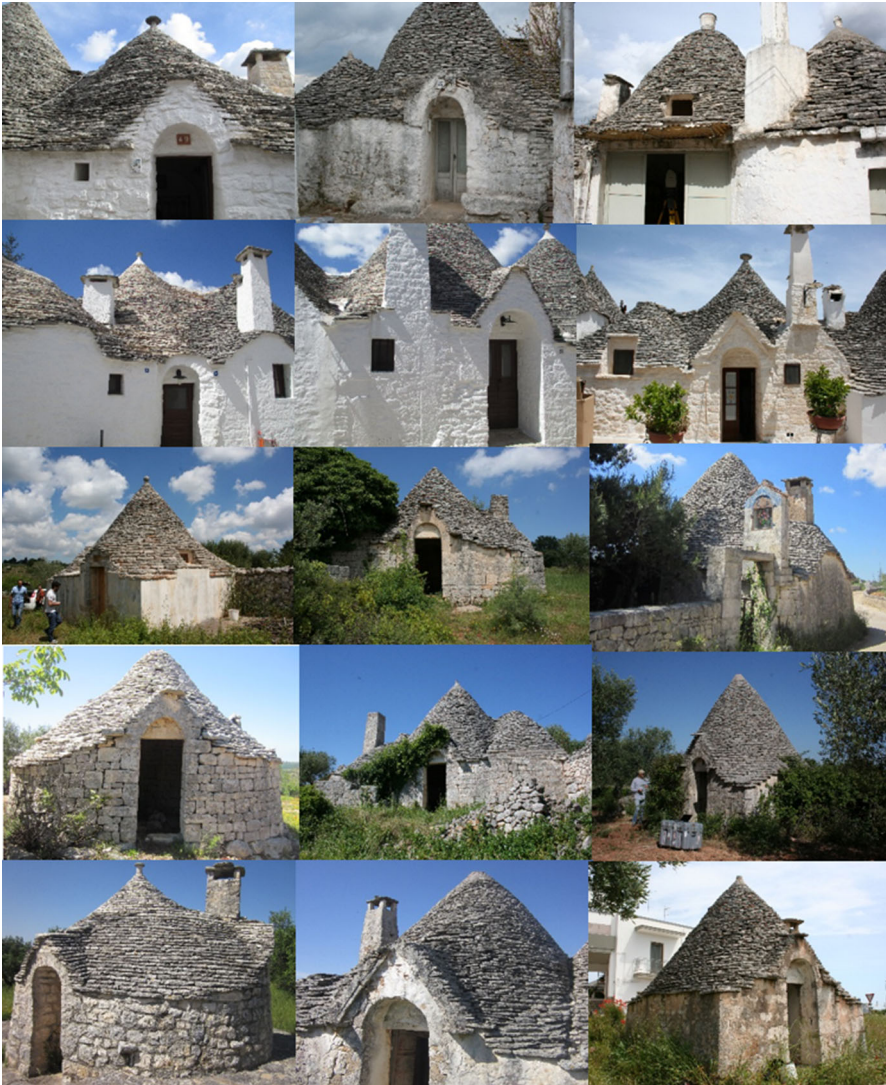
Fig. 3 An overview of the case studies (two of two) considered in the Apuliabase Project. The case studies belong to a wide range in terms of preservation conditions; both well-preserved and crumbling trulli were considered within the city centre (Alberobello) and its countryside
