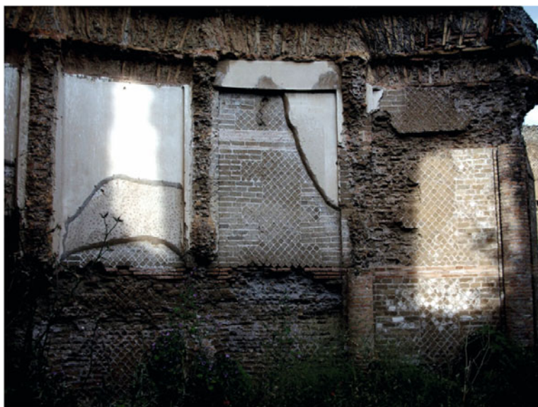
Fig. 13. Accademia, Temple of Apollo, summer solstice 2010. The rectangles of light move towards the right, illuminating panel S12 and the wall of room AC88 (Zooteca) left of the axial door towards AC89. Photo: 20 June at 19:26, by Giuseppe Veneziano
