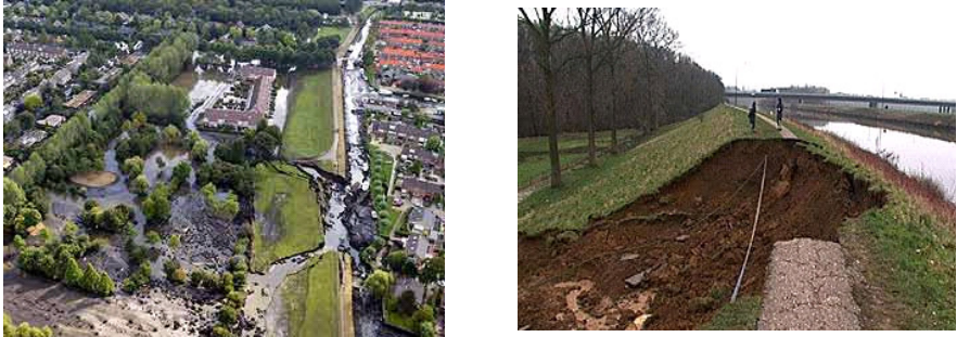
Fig. 1. Water Barriers Under Pressure at Wilnis (left) and Stein (right)
