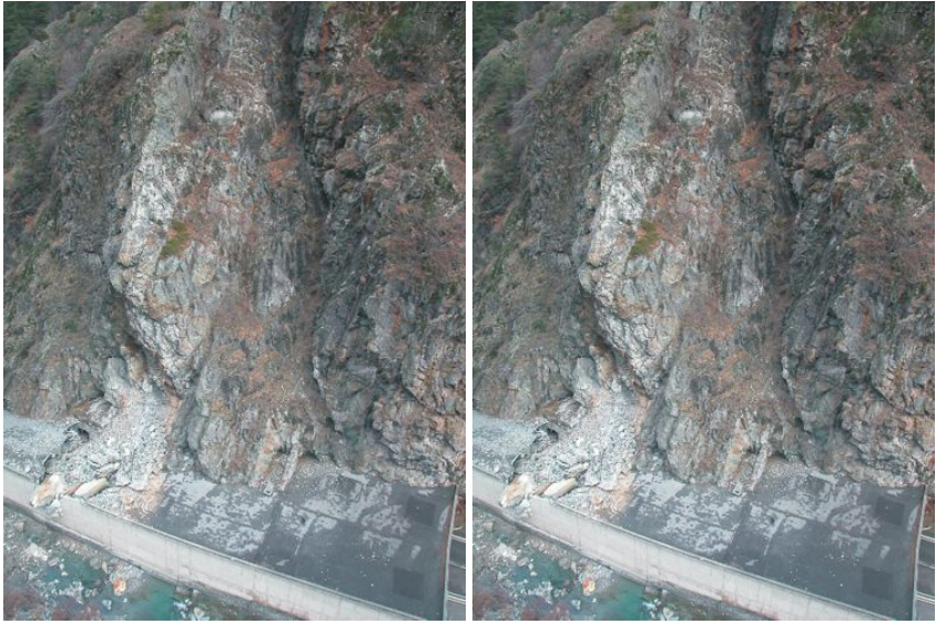
Fig. 5. The Trappistes falaise after the rockslide
