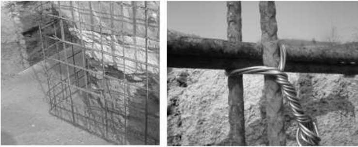
Fig. 5.9. Reinforcing wire at the north-western edge of the field block and overlapping steel mats, tied by twisted wires.
