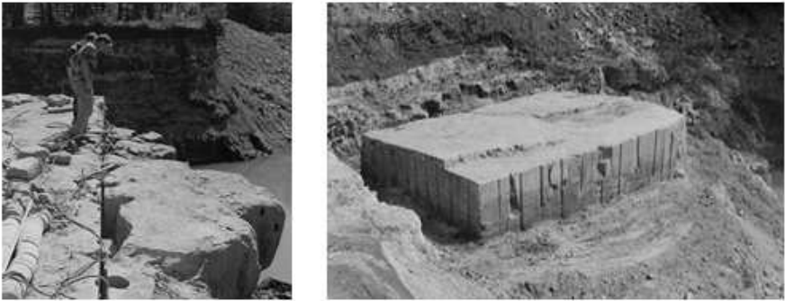
Fig. 5.7. Widening the cutting slots with hydro-pressure cushions (left) while shaping the field block (right); direction of view: south-east.
