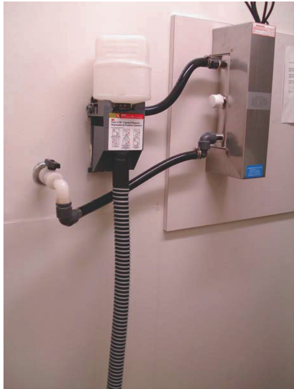
Fig. 12.1 Automatic disinfectant dilution system attached to a UV sterilizer on a water system
