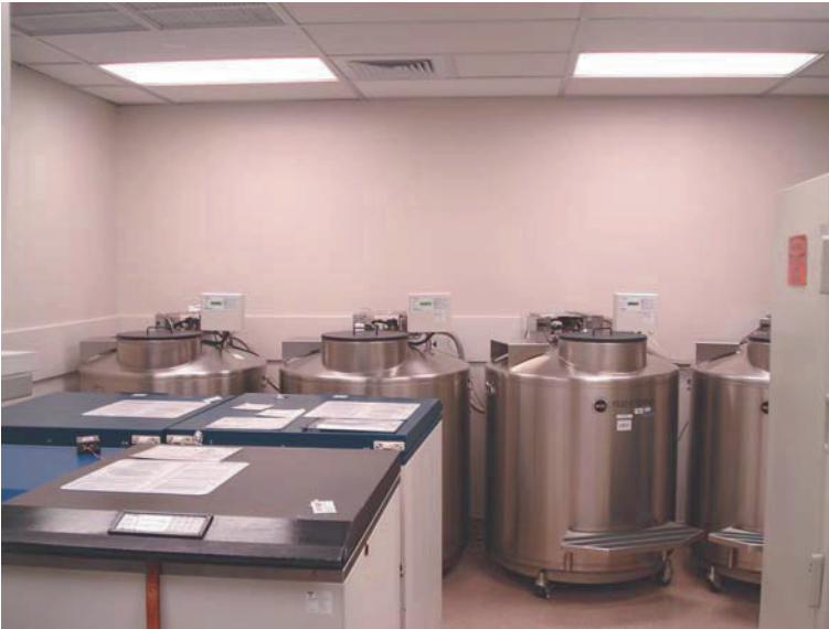
Fig. 6.6 Cell processing facility – nitrogen storage banks
