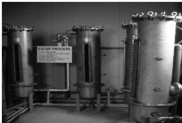
Fig. 2. Pilot plant for phosphorus treatment from farm wastewater.
