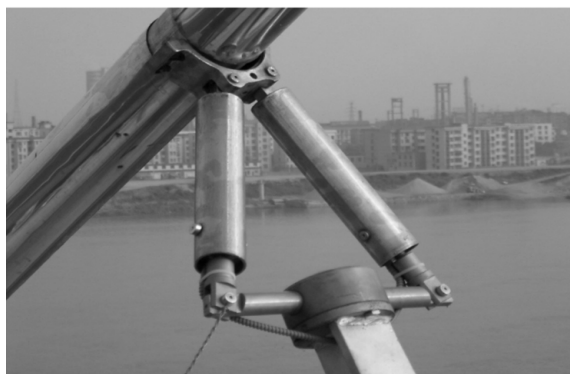
Fig. 25. Full Implementation of MR Dampers in Dongting Lake Bridge
