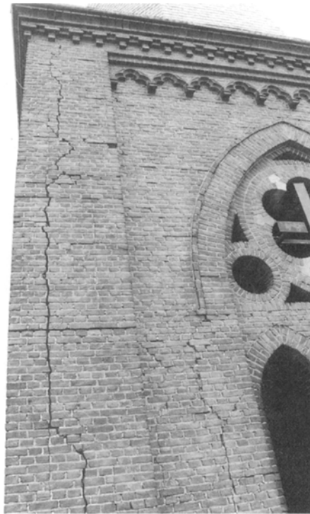
Fig. 1 - Wide (vertical and also horizontal) cracks, on the first sight looking like structural cracks, were found to be caused by swelling compounds in the inner part of the masonry.
