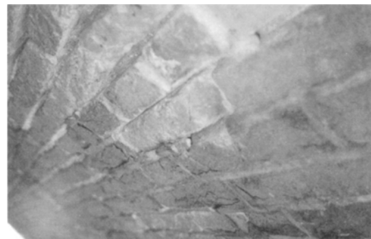
Fig. 2 - Damage in the passage (way) of a historical arch bridge: spalling of brick and pointing is pushed out.
