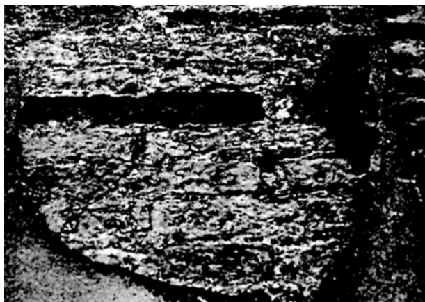
Fig. 3 Deterioration of rendering mortar.
