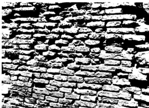
Fig. 2 Deterioration of bricks and jointing mortars.
