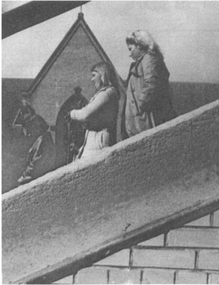
Figure 10. Balustrade of fossiliferous Indiana limestone showing strong corrosion in upper portion by combination of salt fretting by de-icing salt and acid rain attack. Hygroscopic retention leaves the wetline permanently visible. South entrance to Main Building, University of Notre Dame, Indiana.
