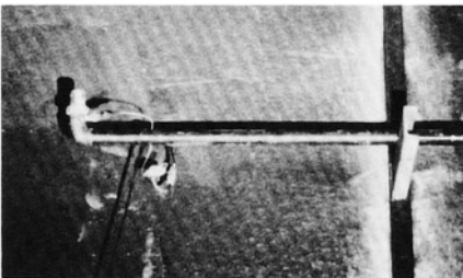
Figure 3. One of the four Halon 1301 discharge nozzles.
