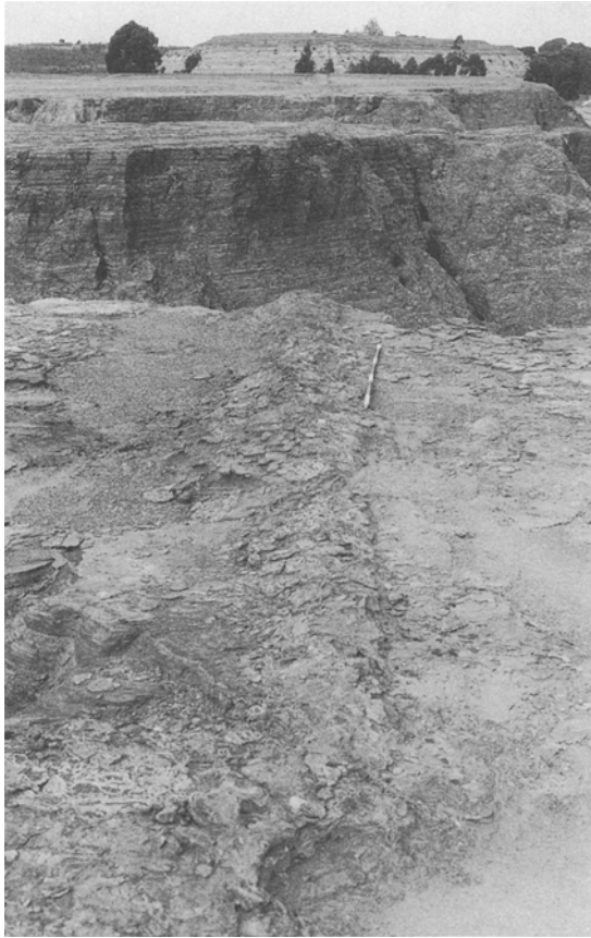
Figure 8. Retaining bund (foreground) built 17 m away from the west wall four days prior to failure in an attempt to reduce the degree of saturation of the area subject to tension crack formation near the west wall (see Table 1).
