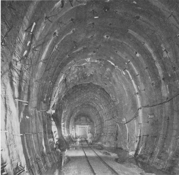
Fig. 10. The elliptical profile in changing rock conditions showing bracing as an emergency measure
