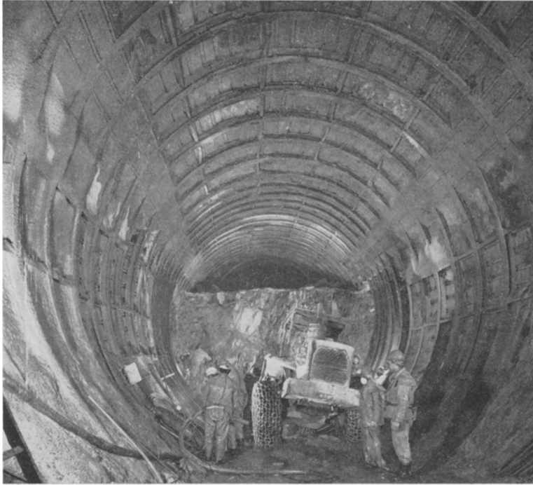
Fig. 14. Heading and bench method of excavation with inner row of steel ribs underpinning upper half
