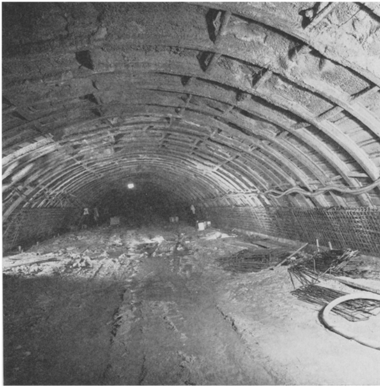
Fig. 13. The top heading with the outer steel ribs and the reinforcement for the longitudinal concrete beam
