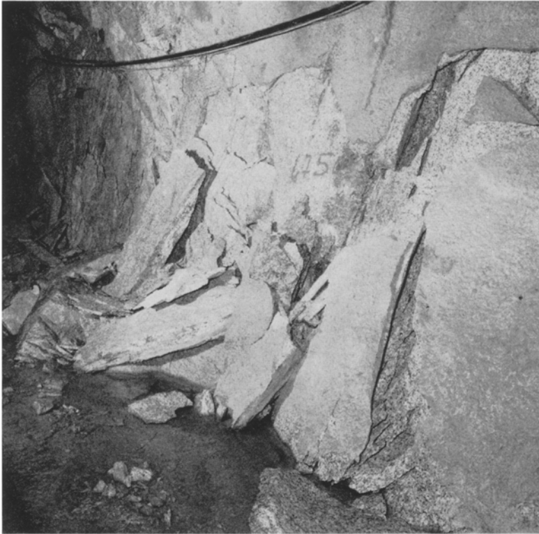
Fig. 8. Spalling of granite
