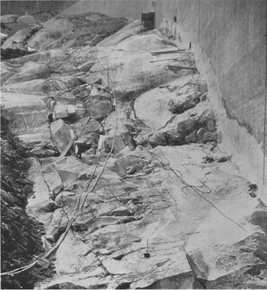
Fig. 12. Longitudinal cracks on the rock surface at the upstream toe of the dam seen after removal of mud
