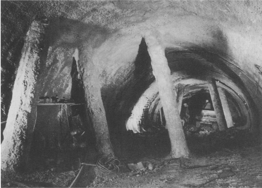
Fig. 19. Tunnel with shotcrete lining traversing the pile group of an underground car park
