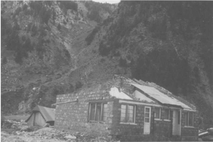
Fig. 7. Heavily damaged restaurant building in the runout zone of 'Rahi' avalanche path (#14 in Figure 2), with the confined track zone visible in the background. Several buildings in this runout are periodically damaged and rebuilt. A mosque and another building were completely destroyed at this site during the 1983–1984 winter.
