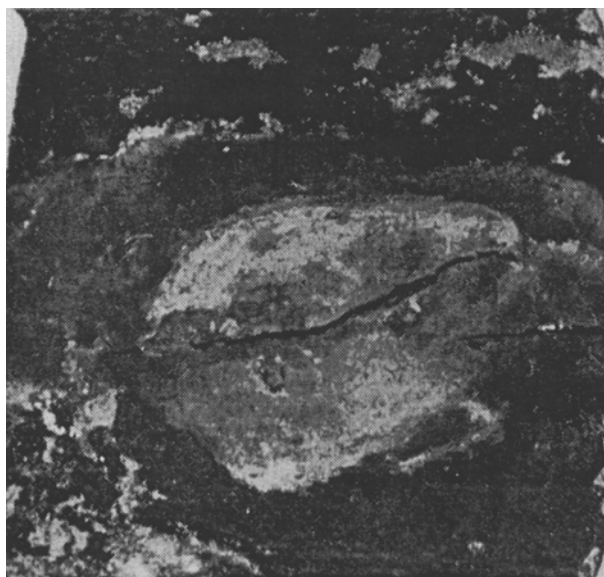
Fig. 2. Typical damage to a steam-generating tube by plastic rupture in the zone of thick multilayer deposits of magnetite.
