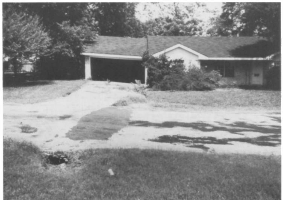
Fig 5 House on Billings Street damaged by 0.4m historical vertical offset across the Long Point fault, Houston, USA (June 1980). Scarp, down to the right, passes through garage and patch in road
