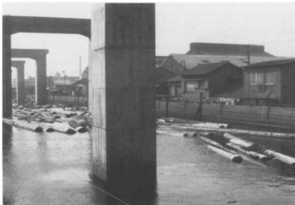
Fig 8 Dike protecting subsided area from inundation by river, Tokyo, Japan (September 1969). River level is at second-floor level of houses. Frames under construction will support roadway over river
