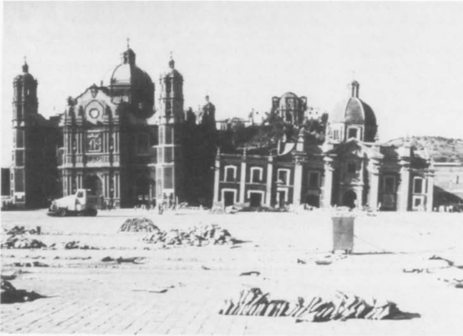
Fig 6 Extreme differential settlement of the Capuchinas Church (right) adjacent to the Basilica of our Lady of Guadalupe, Mexico City, Mexico, caused by weight of the basilica and variable thickness of underlying compressible strata (April 1977)
