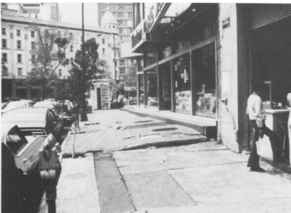
Fig 7 "Rising" building in Mexico City, Mexico (April 1977). Building is built on piles that are founded on firm strata partially beneath compacting interval. Land surface has settled beneath and around building. Note elevated curb of building and buckled sidewalk
