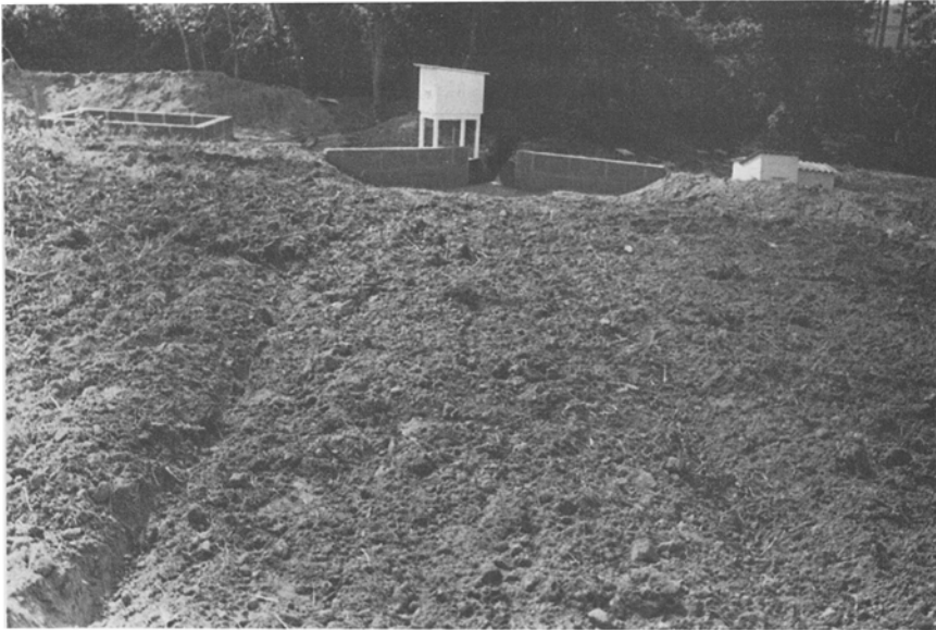
Fig. 1. Runoff and erosion collection system with 1'H-Flume installed within the cement-block retaining walls. Water level recorder is fixed in the white box above the Flume. Sampling tank is housed in the sump on the right.
