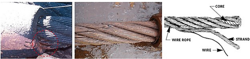
Fig. 2. Broken wires at wire rope endpoint [1].
