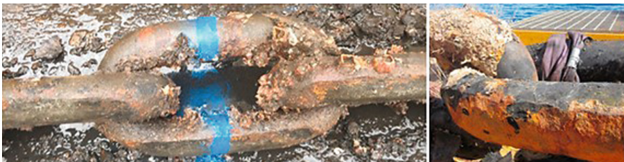
Fig. 5. Ground touching mooring chain with one side material loss [1].
