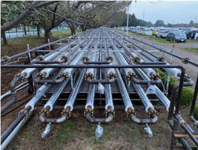
Fig. 14 Main pipes (two sets of 264 pipes of 5.5 m)
