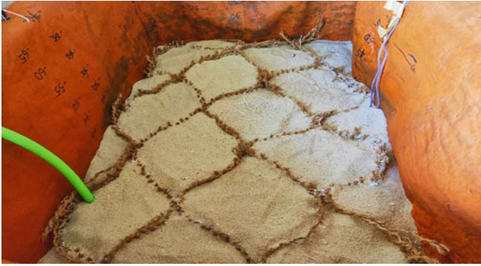
Fig. 3 Placing of coir geocell at the central portion of the test setup
