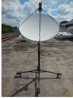
Fig. 11. Reference antenna (dish antenna)
