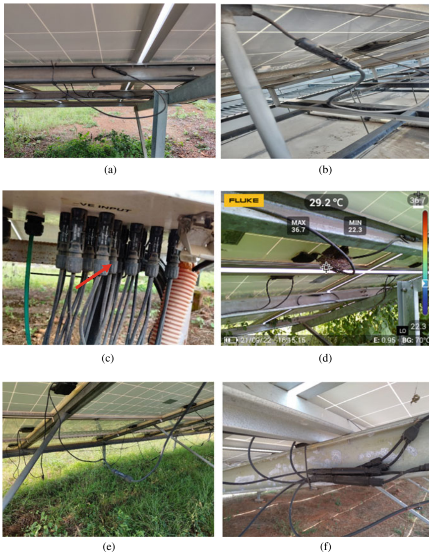
Fig. 4 a Connector hanging on the MMS at Deogarh b connector bend and hanging on rooftop plant site at Delhi c loosely tighten PV plug connectors at SCB marked by an arrow at Pune d hanging connectors and birds nest on MMS e hanging of connectors and wires at Dehradun plant site f connectors bunched together at Chennai site
