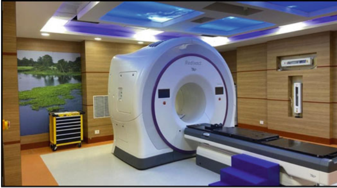
Fig. 1 LINAC treatment unit after installation
