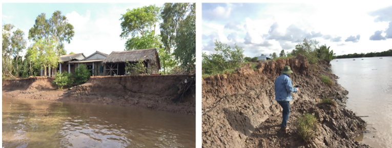
Fig. 6. Bank erosion state at QCB channe
