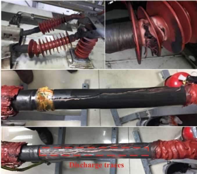
Fig. 1 The faulty cable terminal of high-speed train
