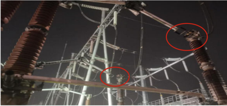
Fig. 2 Photo of DS under incomplete isolating state in the field
