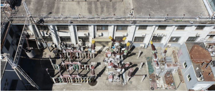
Fig. 2 The overview of the substation
