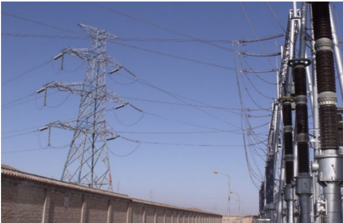
Fig. 1 Picture of incoming conductors of the 750 kV substation
