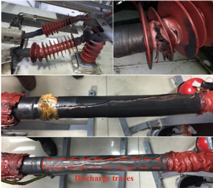
Fig. 1 The faulty cable terminal of high-speed train
