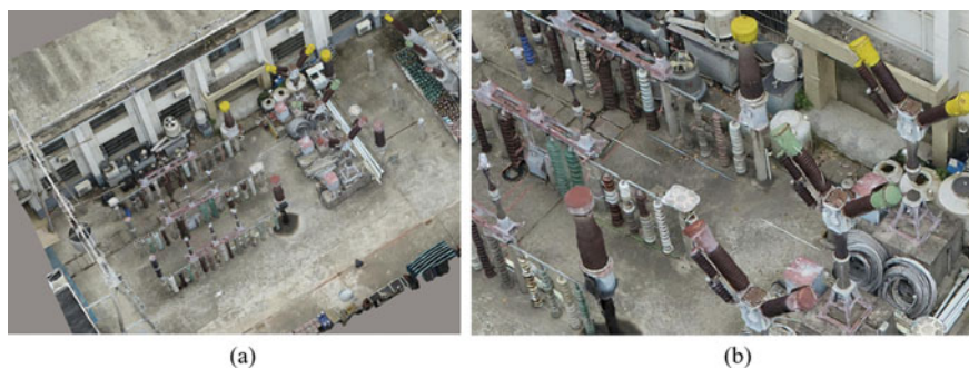
Fig. 6 The 3D model built by the traditional oblique photography method. a 3D model of the substation; b 3D model of electrical equipment
