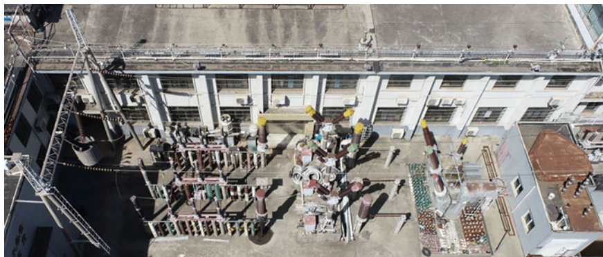
Fig. 3 The overview of the substation
