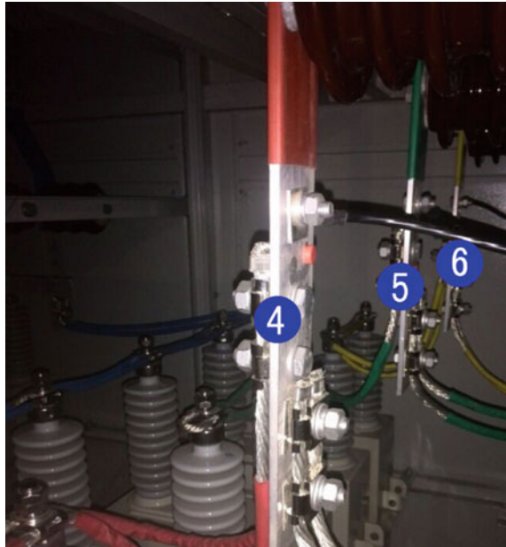
Fig. 7 Test and installation site of the system
