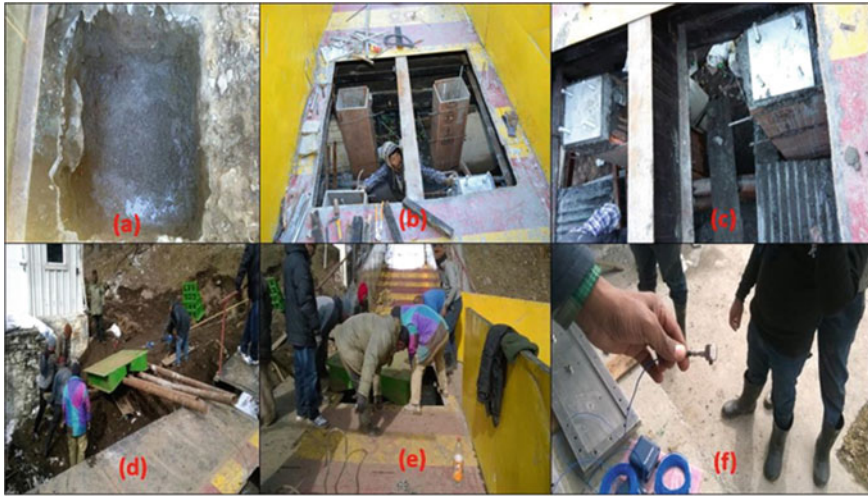
Fig. 3 Installation details of the avalanche impact force measurement system, a foundation, b removal of snow chute sheets and casings, c casting of concrete pillars, d pulling of mild steel base frame, e erection of base frame f inspection of piezoelectric force sensors
