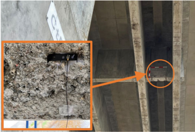
Fig. 1 Example for the damaged RC beam wherein the condition of the support is difficult to investigate
