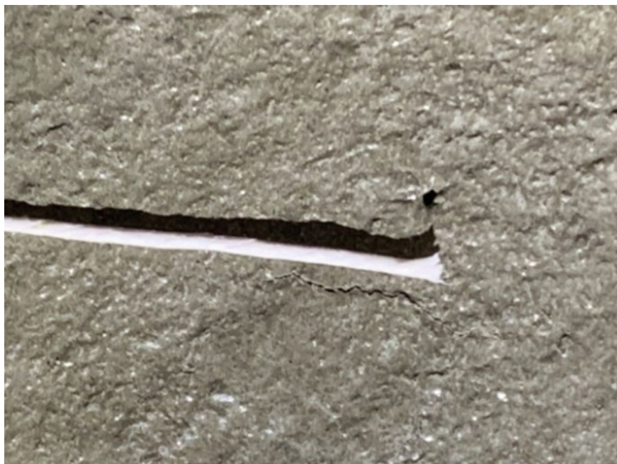
Fig. 6 Plastic shrinkage crack and measuring the length
