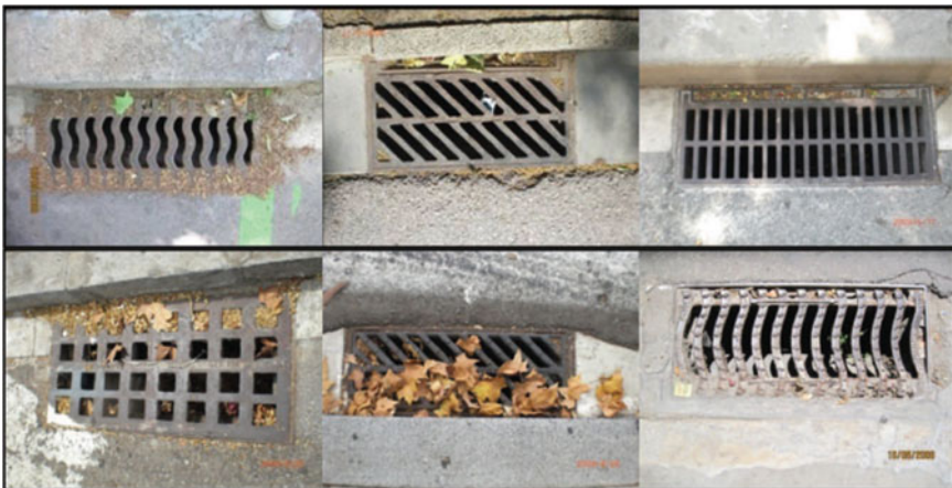
Fig. 3 Grate inlets clogged with debris and tree leaves [21]
