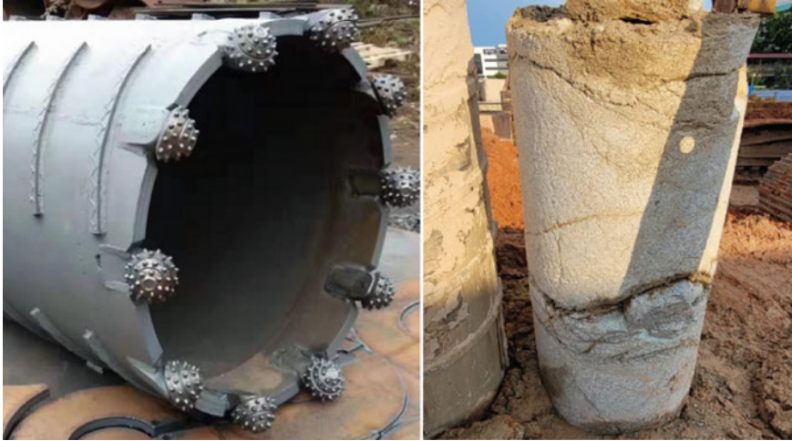
Fig. 1 Core barrel-roller bit and rock core sample by using core barrel-roller bit
