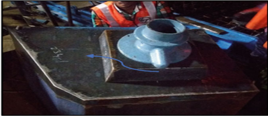
Fig. 4 Wrongly fixed panels
