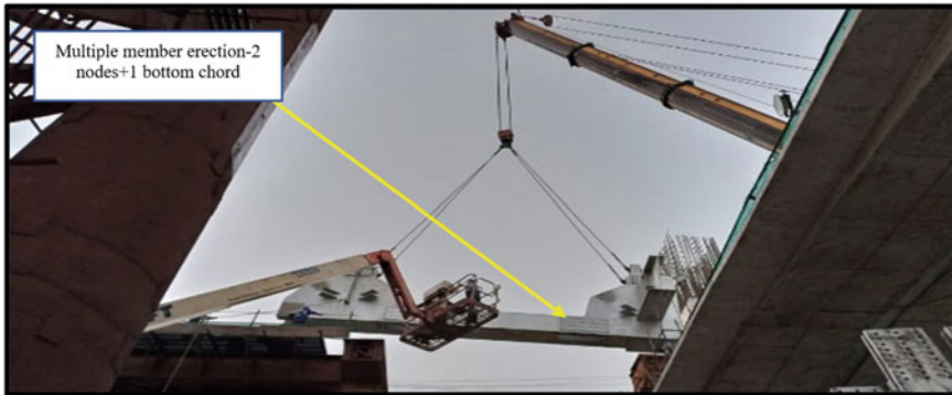
Fig. 10 Erection of multiple members in single lift by 500-ton crane with super lift
