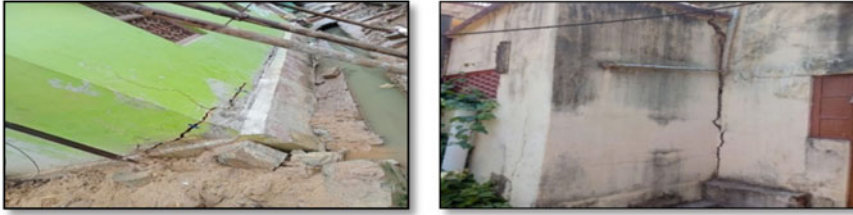
Fig. 1 Building cracks observed during pipe laying by open-cut method (Source L&T Cuttack waste water network project report)
