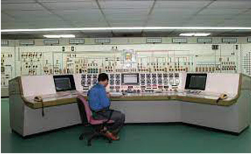
Fig. 1 Control room of Dhruva [10]
