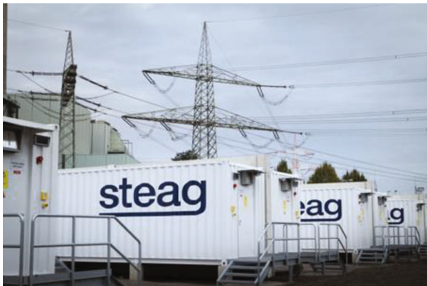
Picture 11.6 6 × 15 MW battery storages of Iqony at power plant sites
