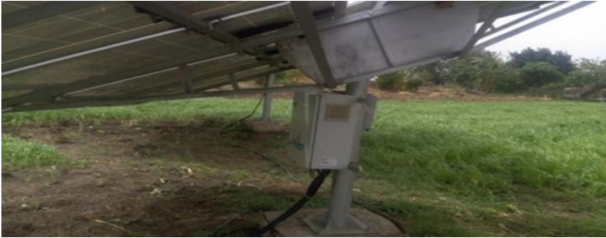
Fig. 4 Controller under solar panel
