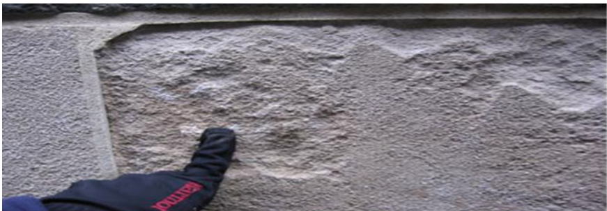
Fig. 13.6 Shows an image of surface loss ( https://vertical-access.com/2015/01/06/material-conditions-series-part-5-surface-loss/ )
