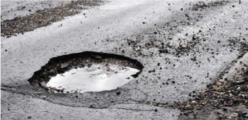
Fig. 13.7 Shows an image of pothole ( https://www.cityworks.com/blog/10-fascinating-facts-about-potholes/ )
