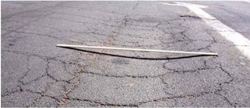
Fig. 13.5 Shows an image of rutting ( https://www.researchgate.net/figure/Rutting-distress-3-The-use-of-reinforcement-in-flexible-pavement-In-order-to-optimize_fig1_321983200 )
