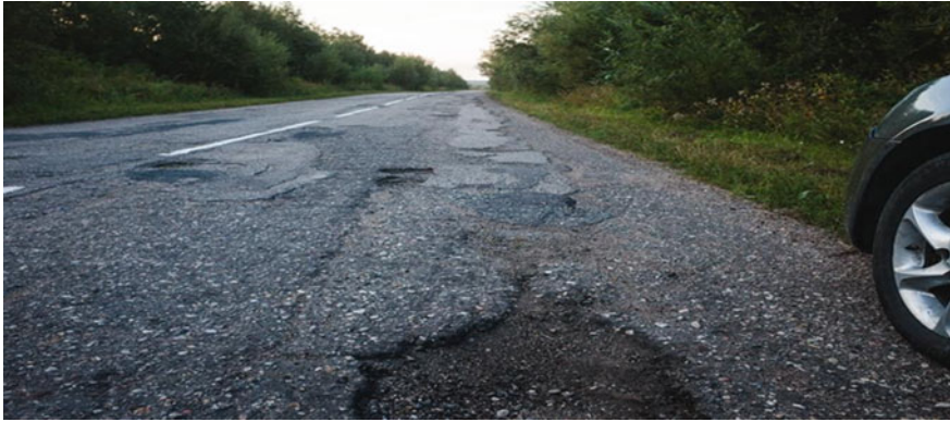
Fig. 13.8 Shows an image of raveling ( https://copavementsolutions.com/asphalt-raveling/ )
