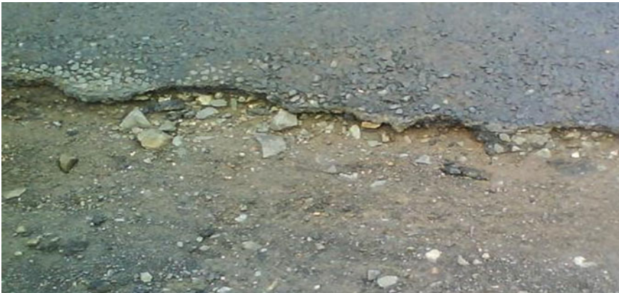
Fig. 13.4 Shows an image of an edge break ( http://lgam.wikidot.com/edge-break )
