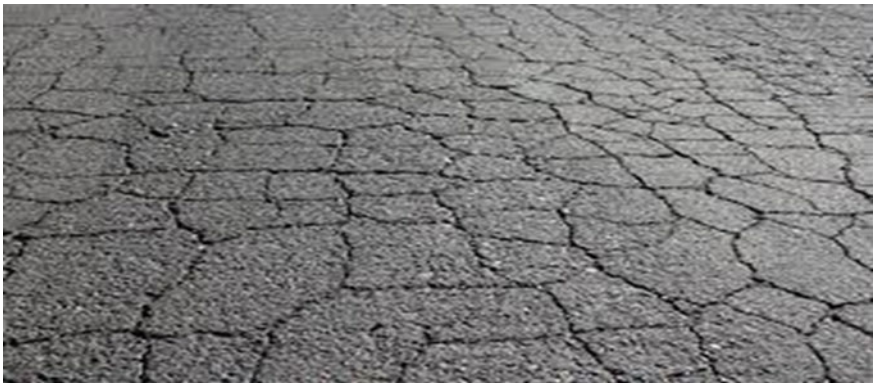
Fig. 13.9 Shows an image of cracking ( https://sableasphalt.com/bad-pavement-cracks-when-crack-sealing-just-wont-cut-it/ )
