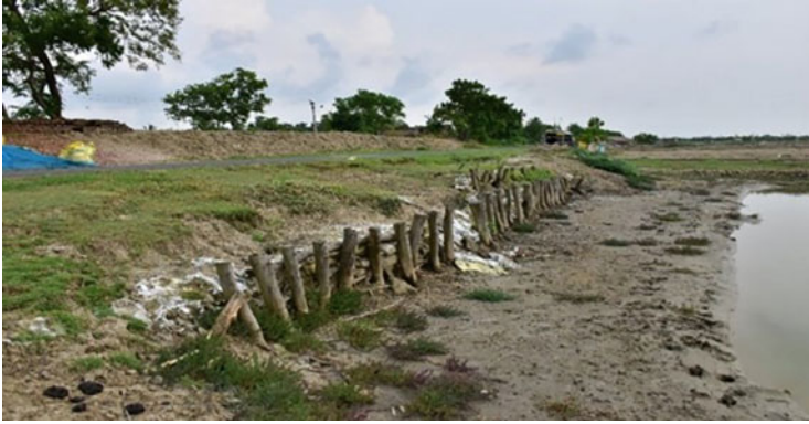
Fig. 20.23 Breach of embankment
