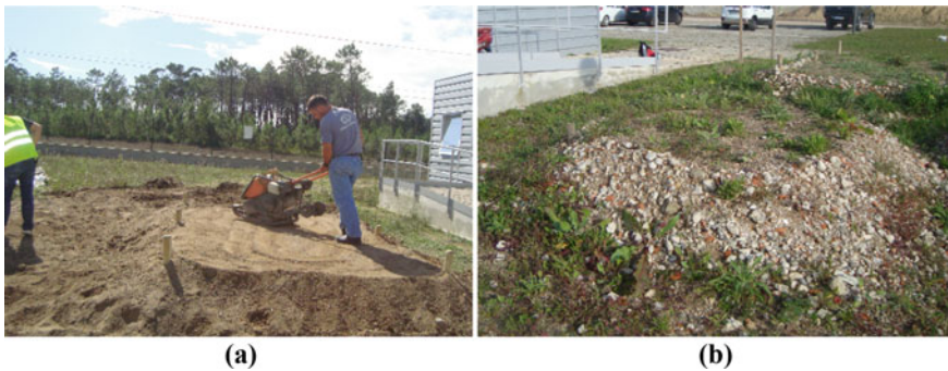
Fig. 2 Small trial embankments: a construction–compaction of the layers; b after 24 months of construction
