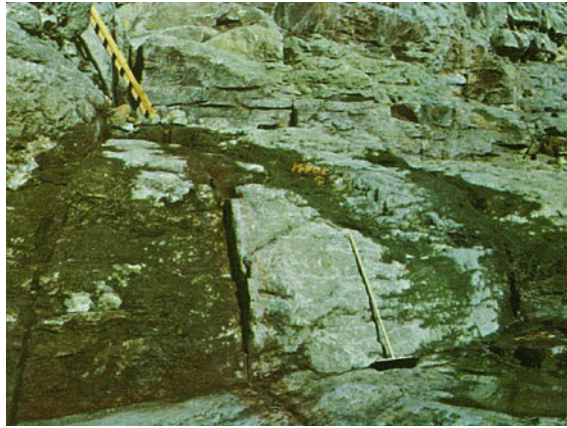
Fig. 2 Vertical joints crossing alignment where grout cap is missing between [11]
