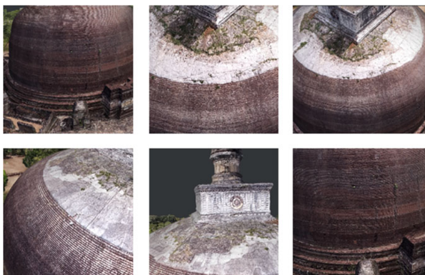
Fig. 13 Brick misalignment and improper keying in the dome
