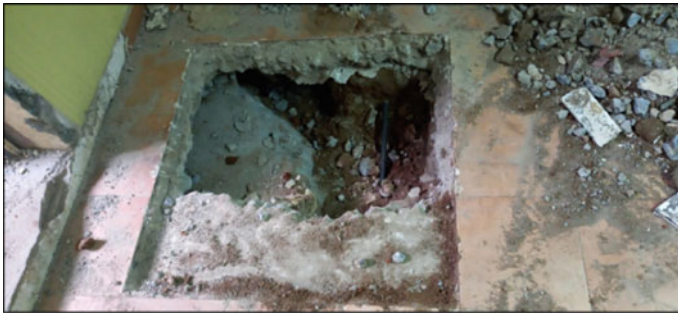
Fig. 21 Mass concrete filling found near footing no. 2
