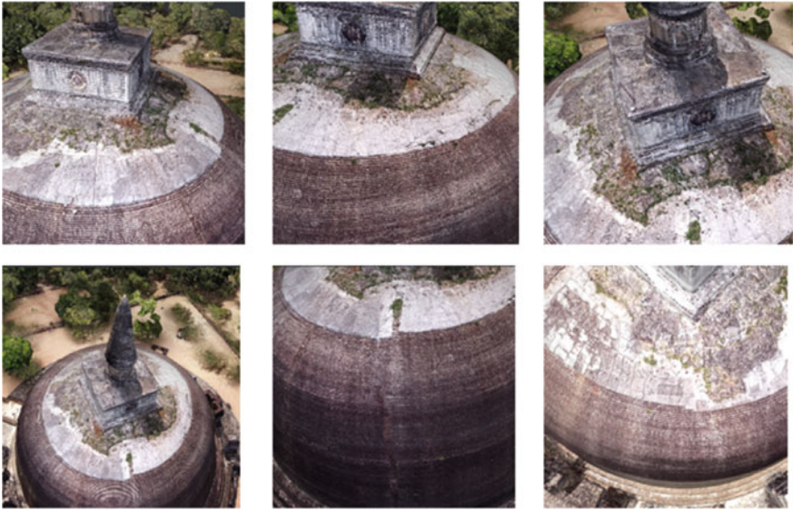
Fig. 14 Cavity and Gully erosion in dome due to water runway
