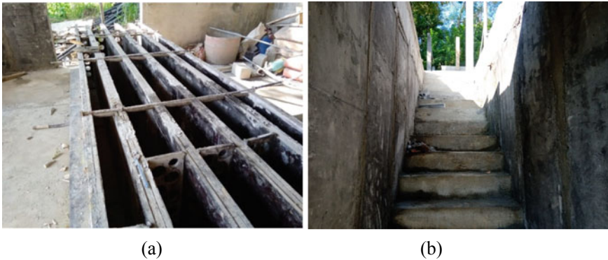
Fig. 4 a Makeshift mould arrangement for producing CLCs and b Assembled wall panels in the case study building
