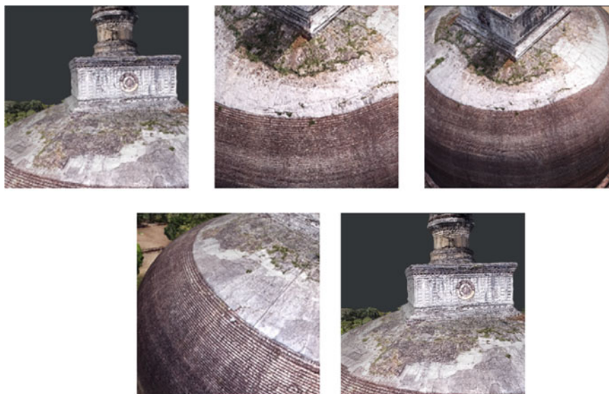
Fig. 12 Delamination of old plaster
