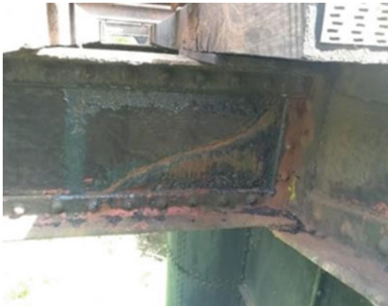
Fig. 3 Crack in rail bearer
