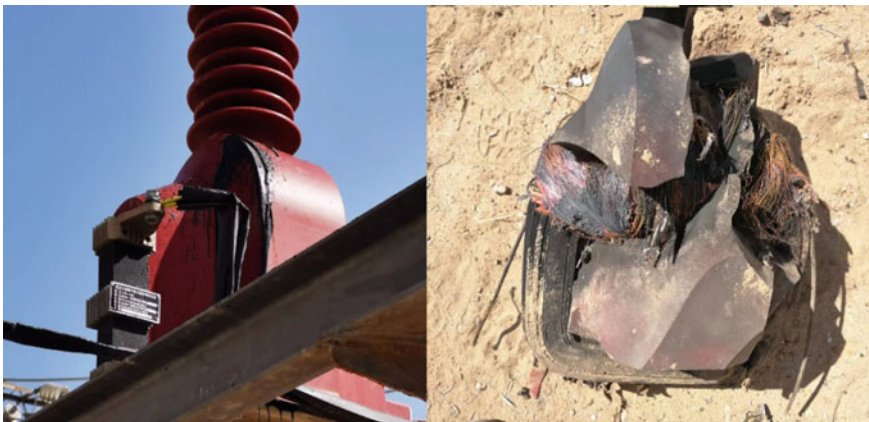
Fig. 6 PT is seriously damaged
