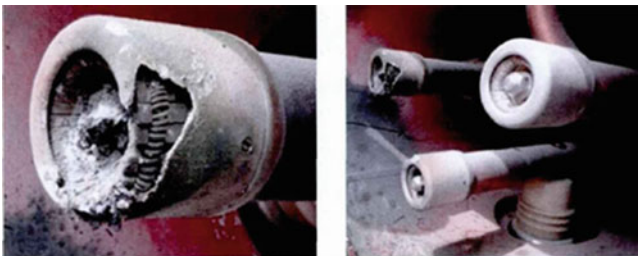
Fig. 2 Overheat failure of busbar joint.
