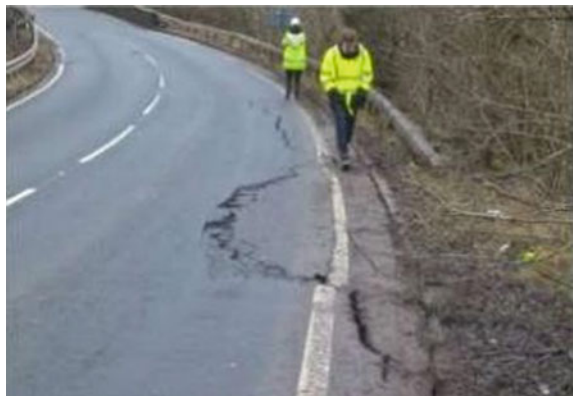
Fig. 1 Cracking appears on the embankment shoulder in road
