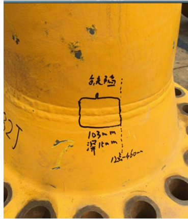
Fig. 5. The defect location
