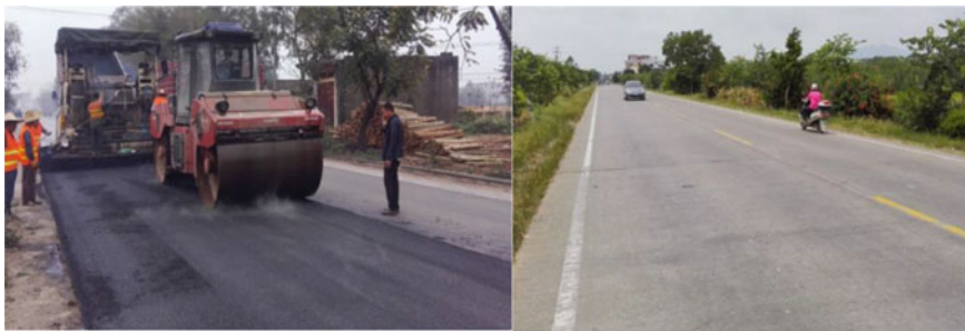
Fig. 8 Comparison diagram of old cement concrete pavement with ultra - thin overlay test section before and after construction
