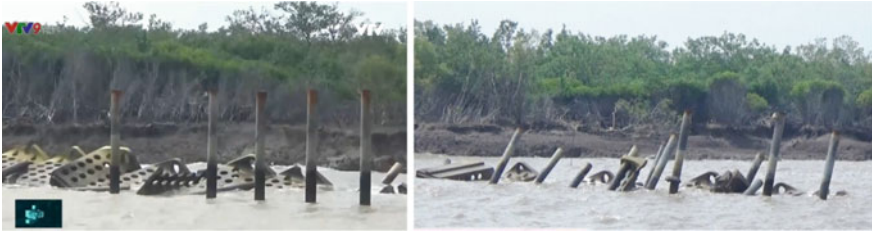
Fig. 24 Reducing wave dike by BUSADCO components in Rach Goc, East Sea of Ca Mau, was destroyed by the storm No. 3 August 2019
