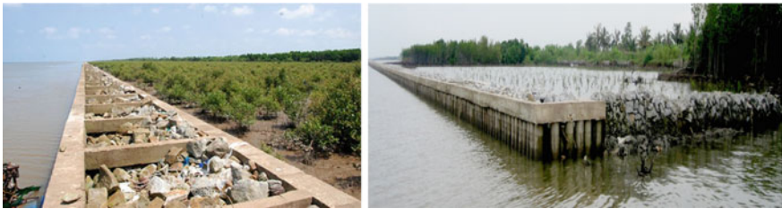
Fig. 15 Spun piles–rock detached breakwaters in the west and east coasts, Ca Mau
