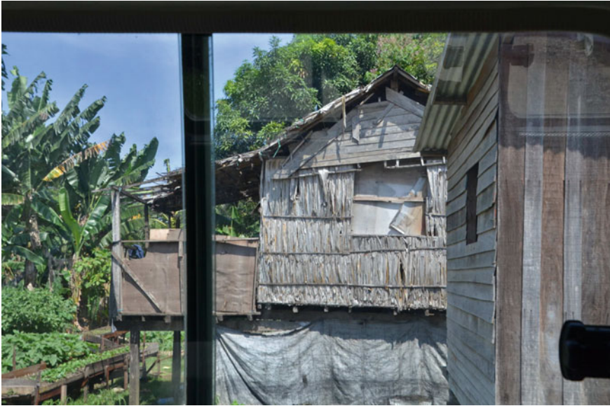
Fig. 4 A mix of materials is used in informal housing in Honiara (Source Tonkin & Taylor)
