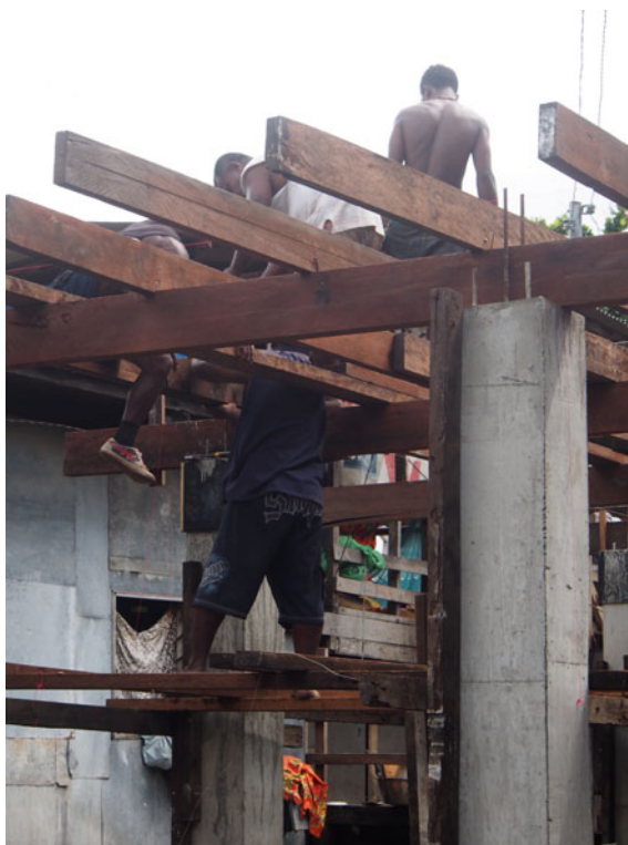
Fig. 5 An informal house raised on concrete posts being built (Source Lianne Marshall)
