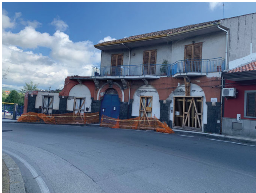
Fig. 7 Semi-destroyed residential building awaiting renovation (Fleri). Source Photo by Iolanda A. Mercatanti (June 2021)
